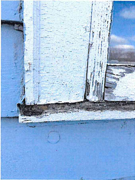
110 8 th Ave S Wood rot
