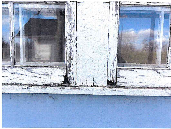
110 8 th Ave S Wood rot
